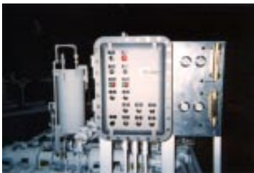
Control Panel of Pump and Filtration Module
