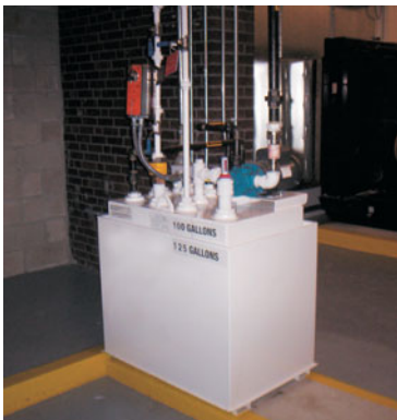
100 Gallon Day Tank with ball valve, overfill protection and Ultra Sonic transmitter for leaks, level readings and a return pump.
