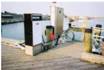
Dispenser mounted on stain- less steel containment pan
