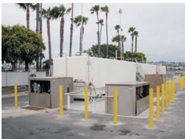
Multiple pumps and dispensers fed the three 12,000 gallon tanks
