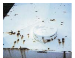
Rust and corrosion on a steel jacketed AST
