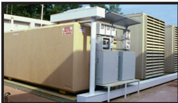
Emergency Power/Boiler Fueling
