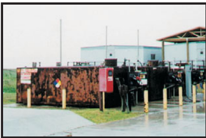
Steel Jacketed Tank In Costal Environment
